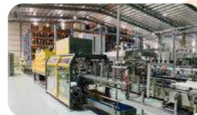
Ceylon Beverages Total Electrical Services
